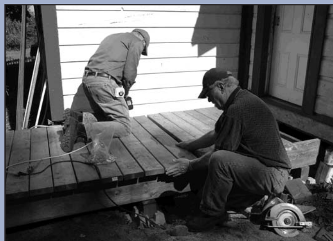
John Fulker and John Woodward building the walkway to Bittancourt Museum's new annex.
